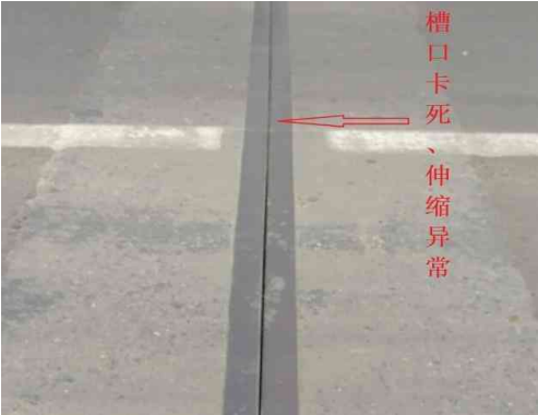
伸缩缝槽口卡死
