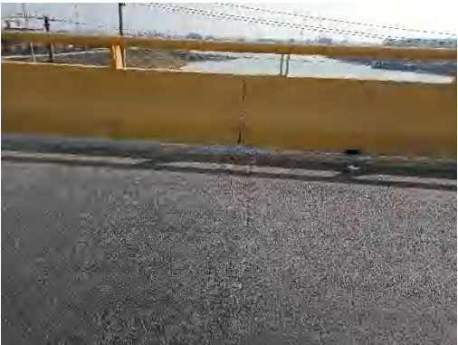
桥面横向裂缝延伸至护栏
