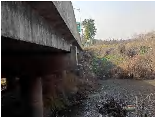
桥墩盖梁剥蚀露筋
