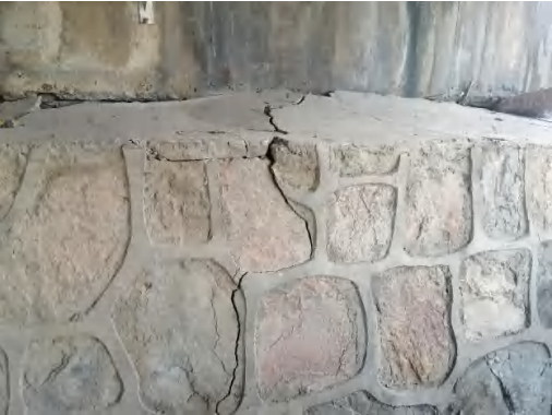
护坡竖向裂缝
