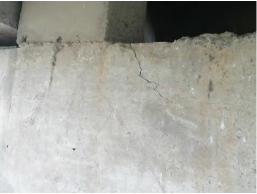
盖梁顶斜向裂缝
