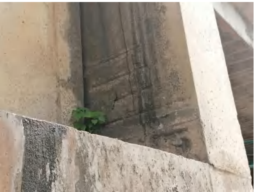
桥台盖梁渗水钢筋锈胀
